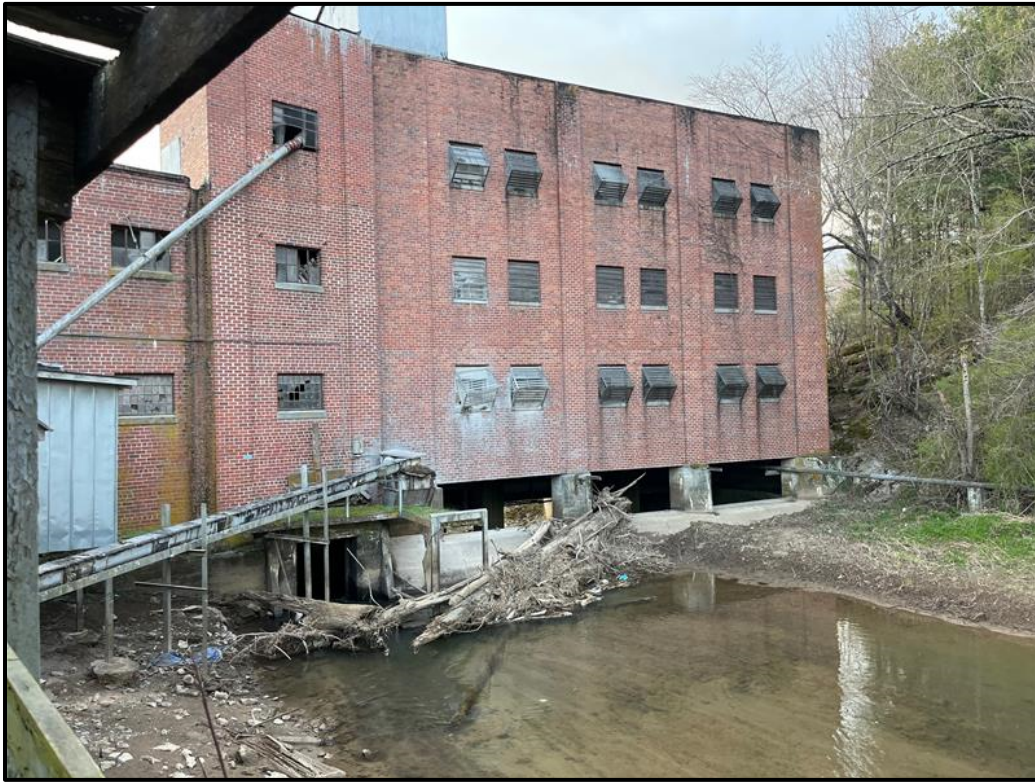
Figure 71: Mill Building March 2023 capturing debris
